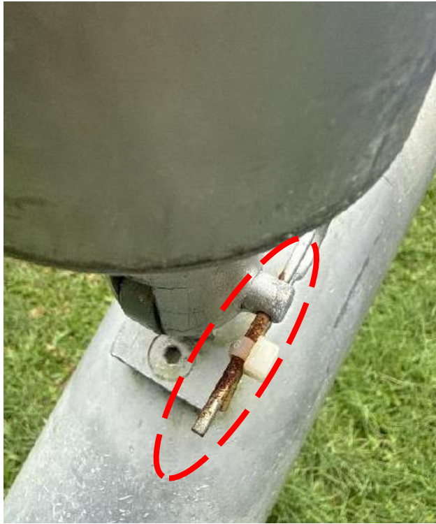
Corrosion at structural components
