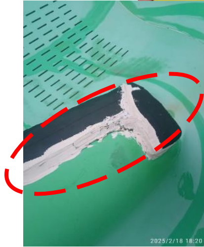
Worn flume surfaces
