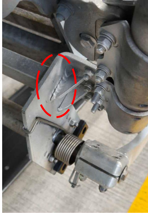
Cracks found on welded area
